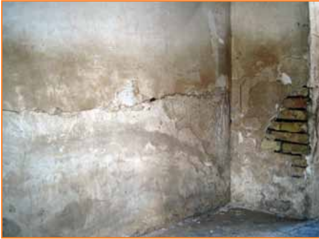
Fig. 3. Damage caused by water seepage on the SW wall, adjacent to B1-1/3 building
