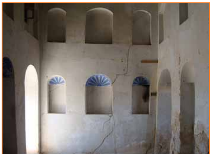
Fig. 2. Example of crack pattern of damaged structures
