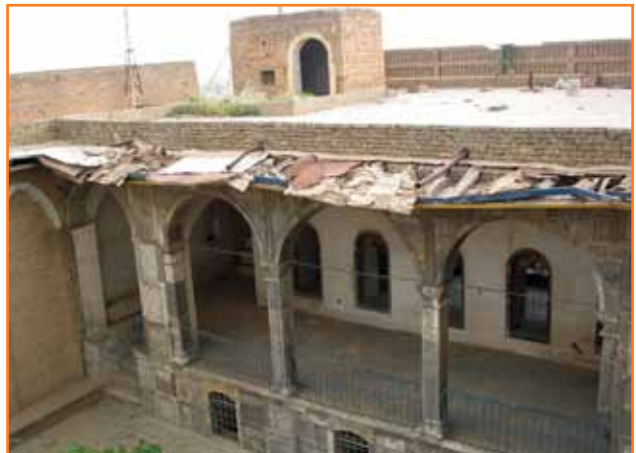
Fig. 2. Façade, NNW prospect (view from the roof). Degradation of wooden shed
