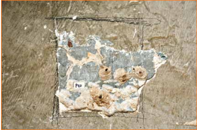
Fig. 2. Stratigraphic test in the SW room, south wall. Note the green painting of the phase 1
